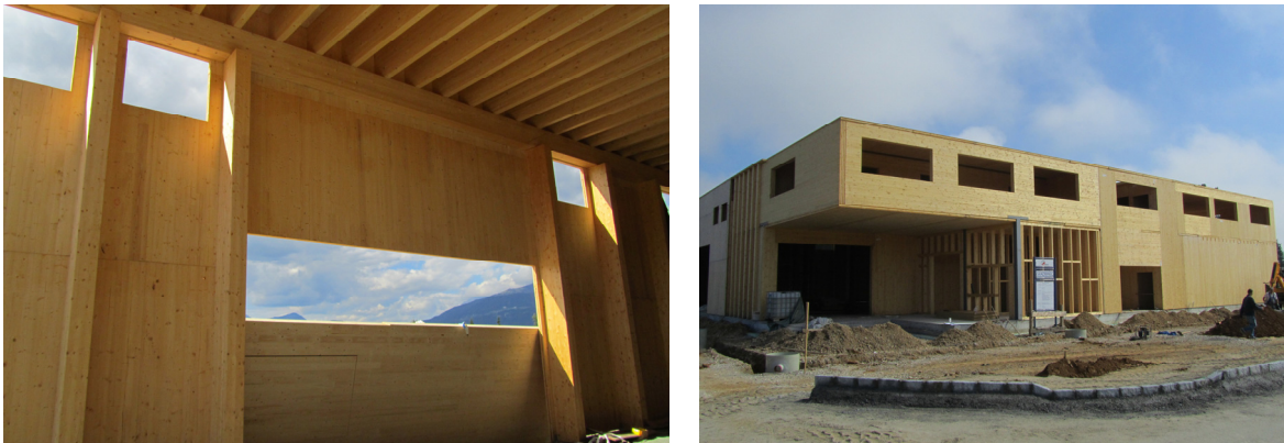
Fig 1: Ekoprodukt storage hall. Bracing system (left), cantilever (under construction) on the right.
